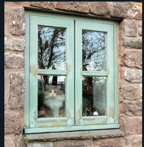
Old, flaking timber windows in need of updating and replacing.
